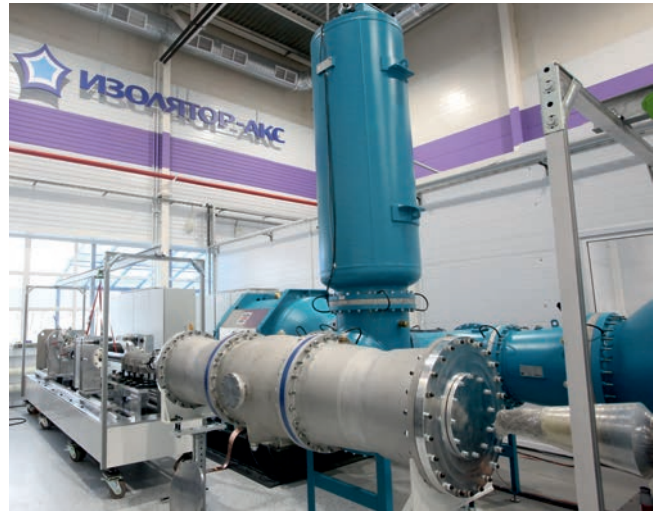
Laboratory for acceptance testing of cable accessories
