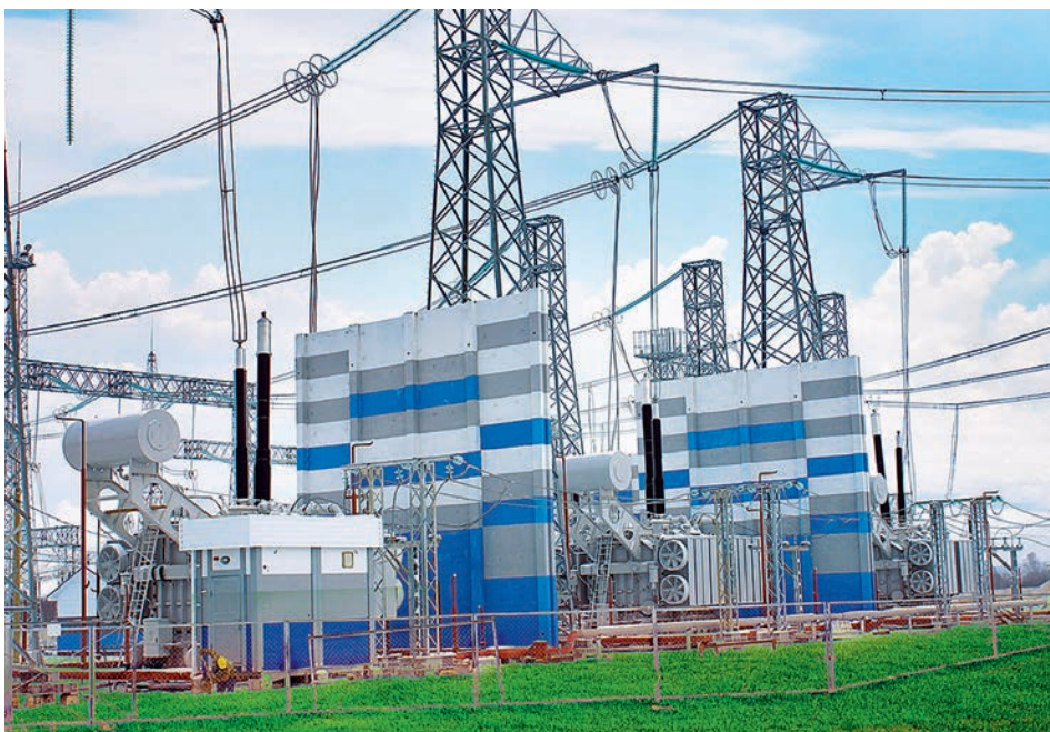
A group of 750 kV single-phase power autotransformers with 1251 MVA rated power at the 750 kV Gribovo substation of the Main Power Systems of Center, one of the substations of the power distribution scheme of power unit 4 of the Kalininskaya NPP (photo: Rosseti FGC UES)
