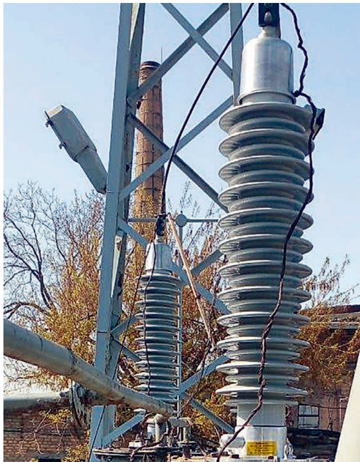
The 126 kV Izolyator RIP bushings installed on the transformer of Uzskabel substation instead of outdated counterparts
