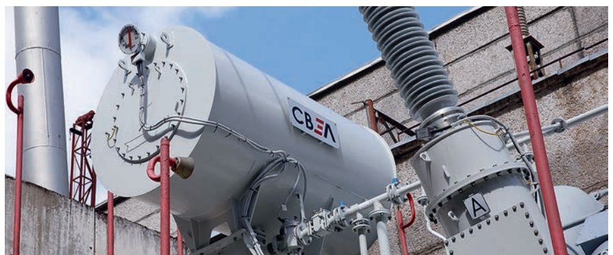
A 220 kV SVEL power transformer, equipped with Izolyator high-voltage bushings
