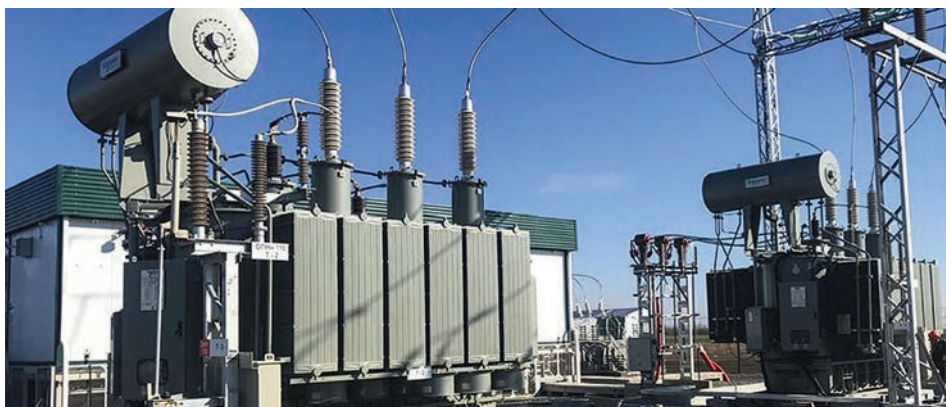
Power transformer equipped with Izolyator high-voltage bushings as part of a 110 kV complete transformer substation manufactured by Electroshield Samara
