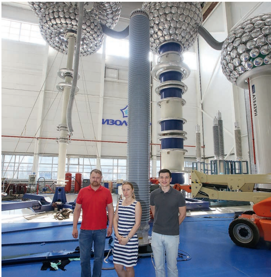
Inspection of tests of Izolyator high-voltage bushings is carried out by the Leading Engineer of the Leningrad NPP-2 Dmitry Kruglov (R) and the Leading Expert of VO Bezopasnost Victoria Goryachaya
