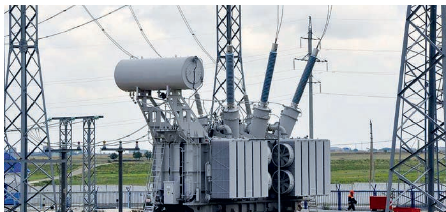
Transformer with Izolyator HV bushings at 330 kV substation Artyom of MPS South
