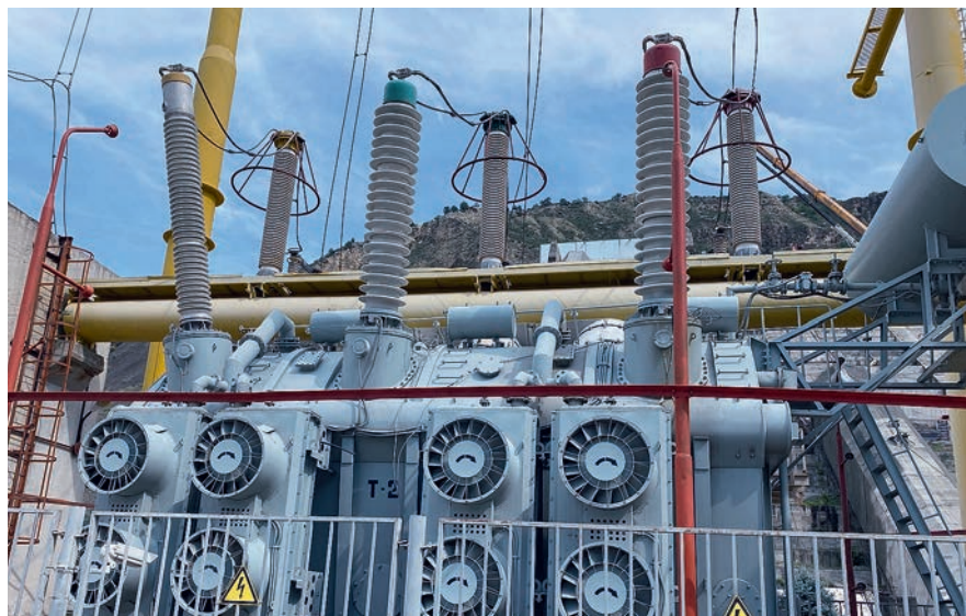
A 330 kV transformer with Izolyator high-voltage bushings at the Irganayskaya HPP of the Dagestan branch of the RusHydro Group
