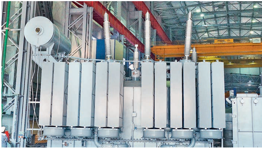
A 250 MVA PMTT transformer with Izolyator high-voltage bushings manufactured for FGC UES (photo: energybase.ru)
