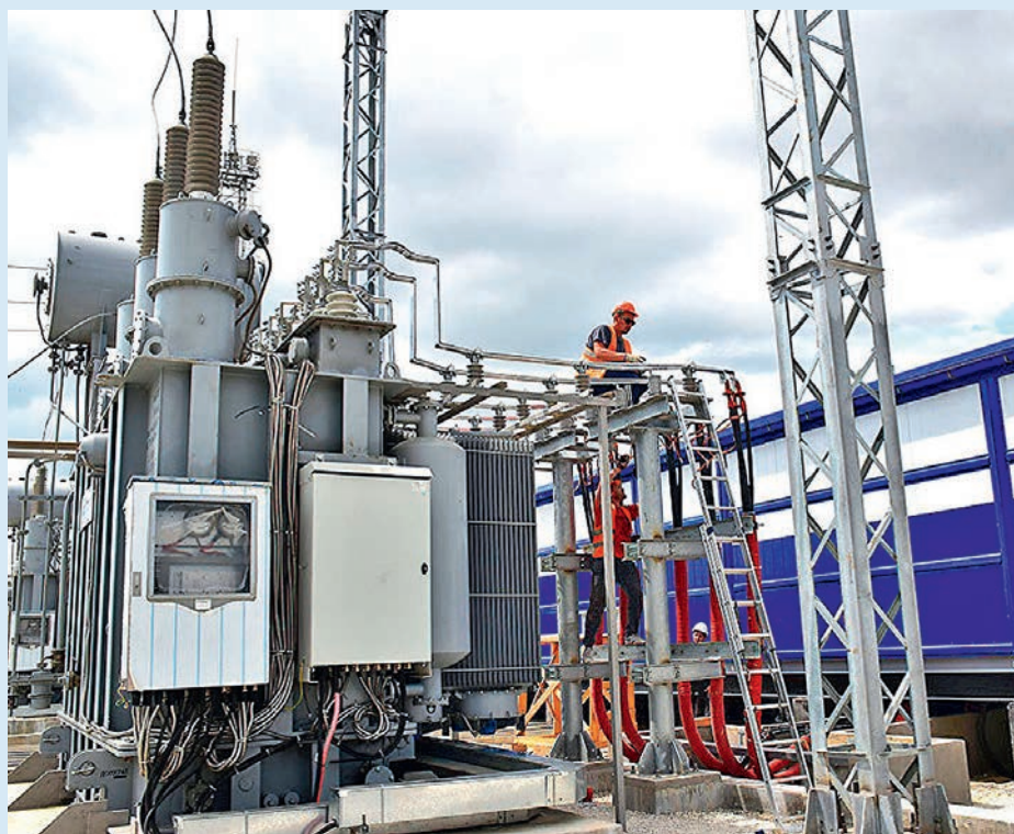
110 kV Airport substation of Krymenergo. Izolyator bushings are installed on the transformer (photo: Krymenergo)
