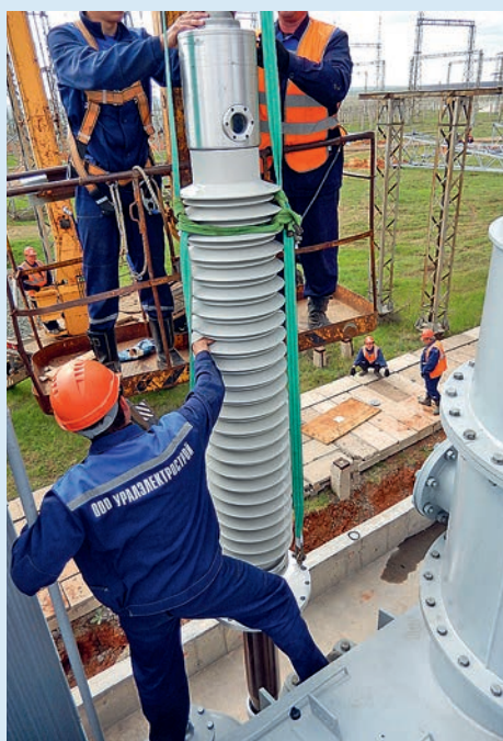
Installation of a 220 kV Izolyator bushing with internal RIP-insulation in an autotransformer of the MPS Ural
