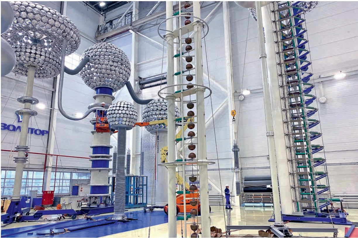
Test Center of Izolyator plant
