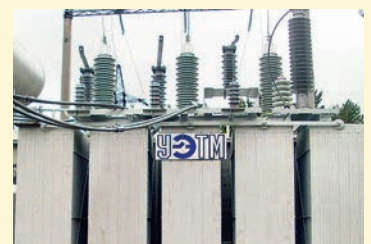
A 110 kV Uralelectrotyazhmash oil power transformer with Izolyator high-voltage bushings (photo: Uralelectrotyazhmash)
