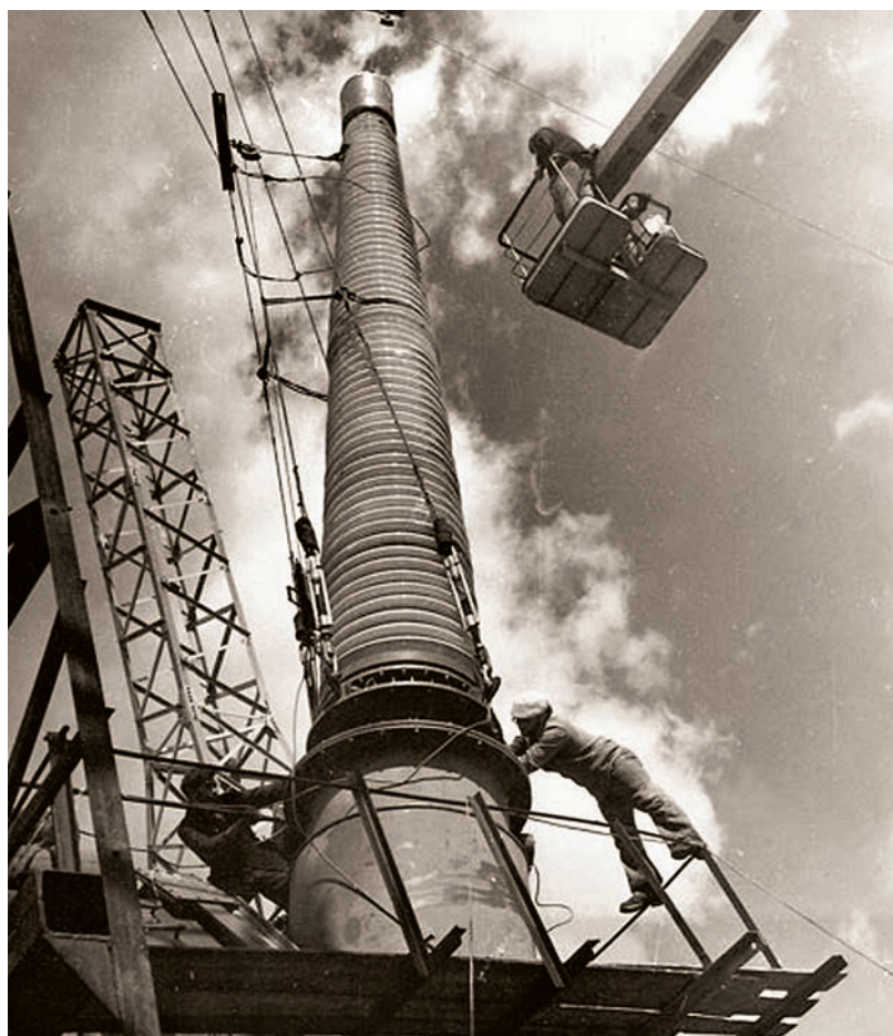
Installation of 1150 kV bushings on the power equipment of the Ekibastuz-Kokchetav-Kustanay power line in the 1980s
