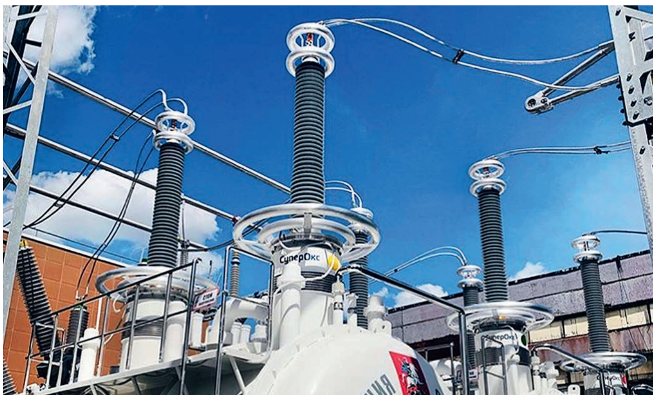
220 kV Izolyator RIN bushings on a superconductive current limiter by SuperOx, installed in the electric substation Mnevniki in Moscow
