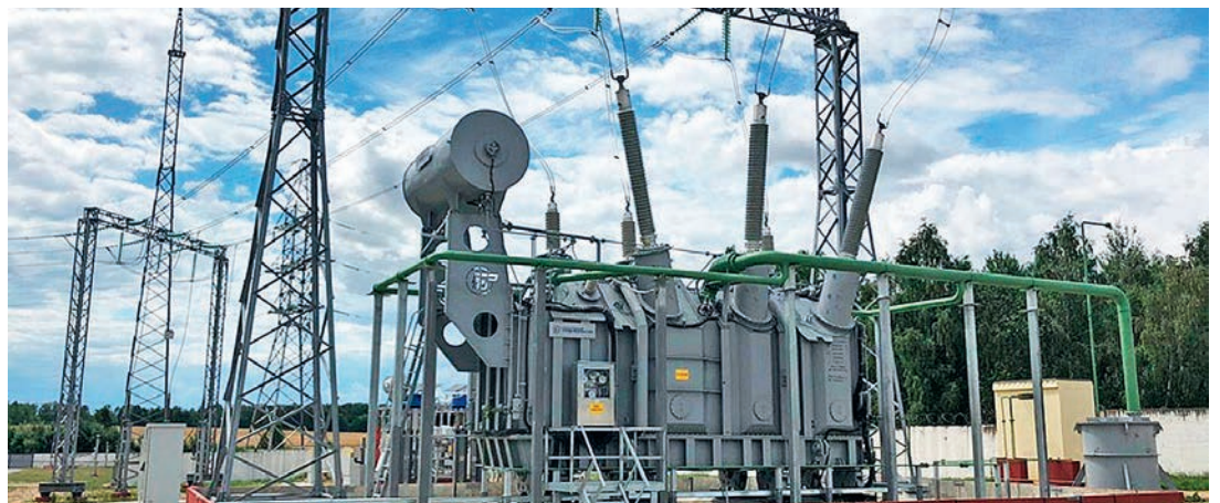
A 200 MVA autotransformer with Izolyator HV bushings at the 330 kV Baranovichi substation in Belarus
