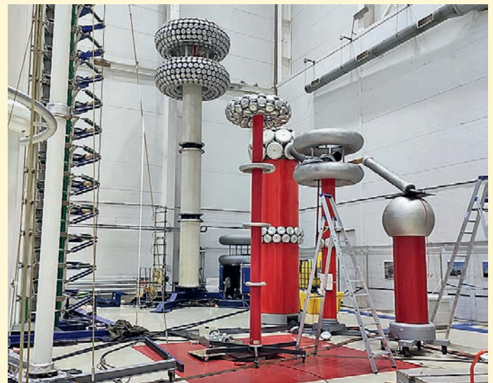
Verification of a 750 kV voltage class calibration divider at the Izolyator test center
