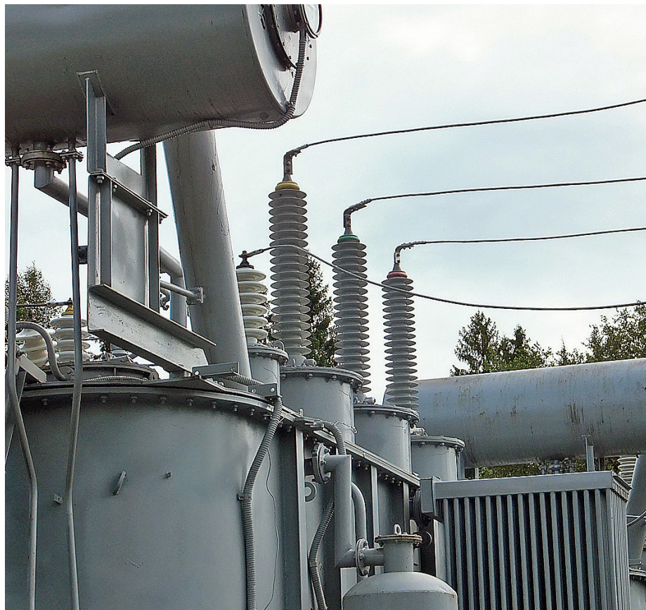
110 kV Izolyator bushings on a transformer
