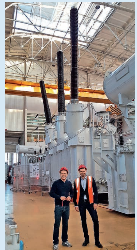
Purchasing manager at SVEL plant Danila Safin (L) and Maxim Zagrebin at SVEL – Power Transformers in Ekaterinburg. At the background – a 265 MVA transformer with 550 kV Izolyator bushings, made for RushHydro Group
