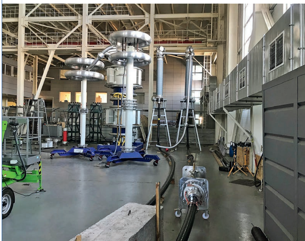
Acceptance tests of a 220 kV IKM-245 external end sleeve in the All-Russian Research, Design and Technology Institute of The Cable Industry Test Center in Podolsk
