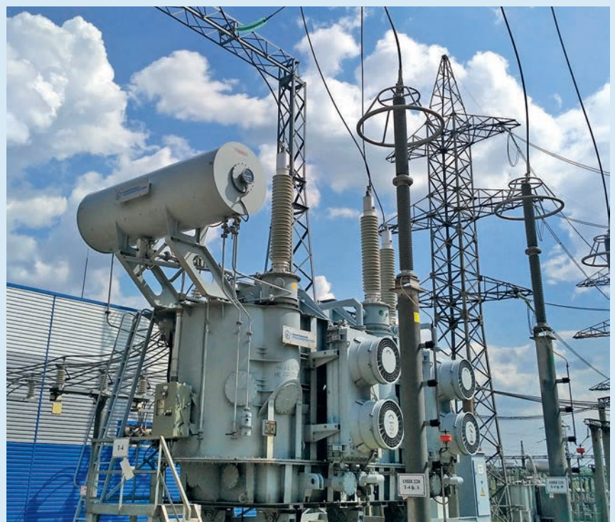
Transformer with Izolyator HV bushings at 500 kV Kurdyum substation of MPS Volga
