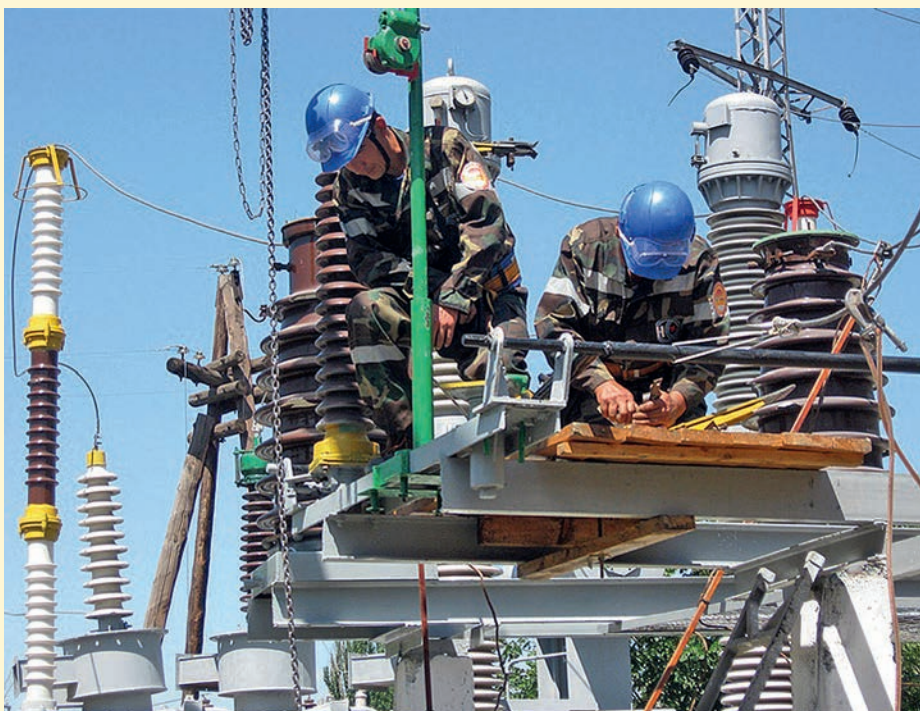
Photo: National Power Grid of Kyrgyzstan
