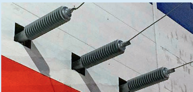
126 kV Izolyator wall bushings, installed in a wall of the closed-type switch gear of 110/10 kV S/S Beregovaya of Chukotenergo
