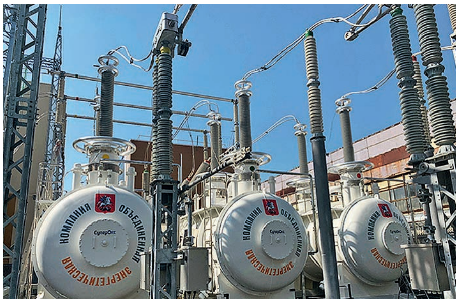
SuperOx high-temperature superconducting current limiter with Izolyator high-voltage bushings at the Mnevnik electric substation of the United Energy Company in Moscow (photo: United Energy Company)
