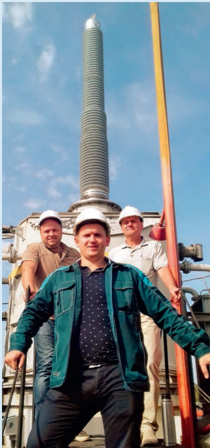
Installation of the first 750 kV bushing with RIP-insulation in Belarus, manufactured by Izolyator, L-R: Dmitry Mashinistov, Anatoly Tereshchuk, leading engineer of Riko representative office in Belarus and Vyacheslav Maskalik, head of the 750kV «Belorusskaya» substation
