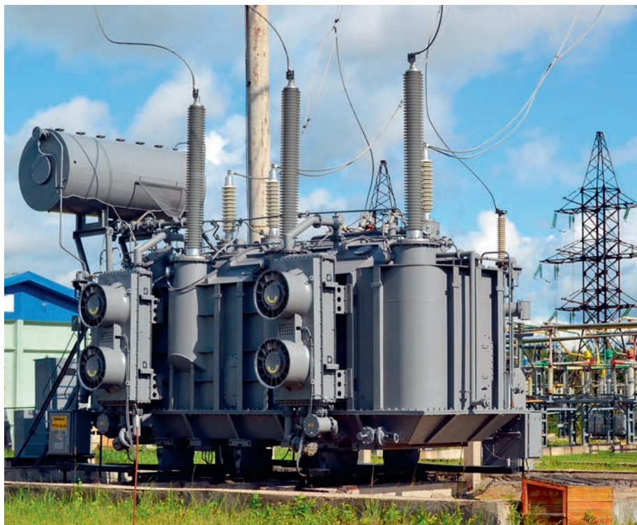
Isolator bushings of 220 and 110 kV voltage classes at the transformer of the FGC UES substation
