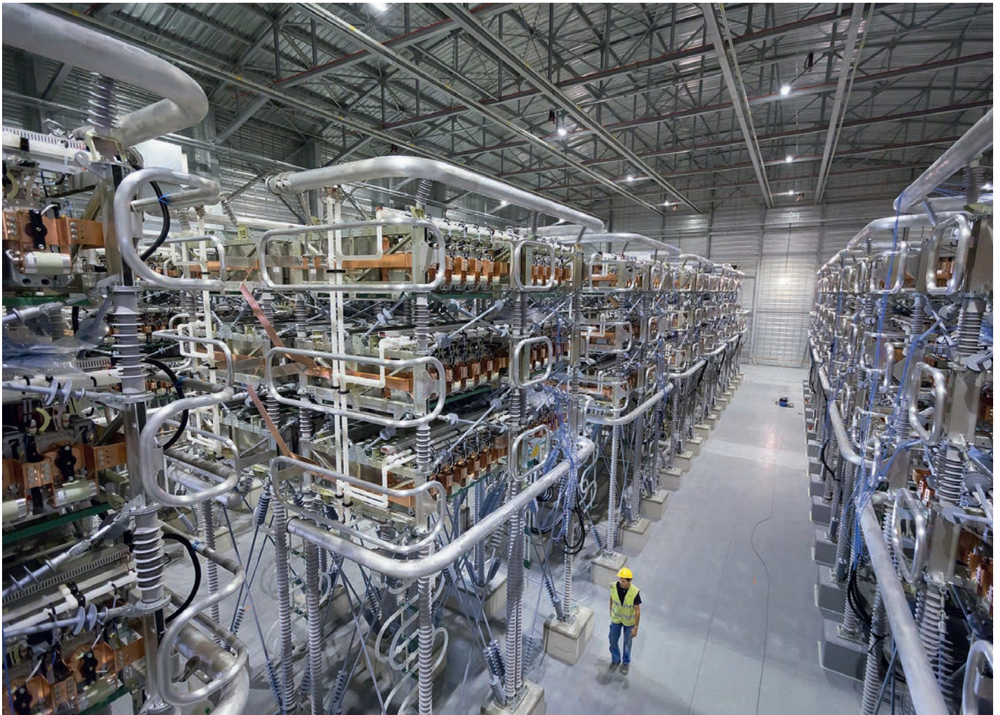
Rectifying equipment shop for direct current transmission between France and Spain. 1000 MW capacity on IGBT
