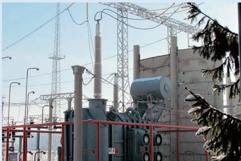
220 and 500 kV Izolyator bushings on a transformer of the FGC UES substation
