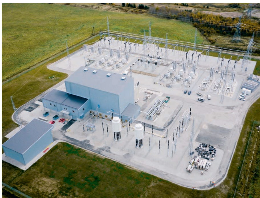
Converter substation of direct current transmission Estlink 2 (Estonia - Finland). Capacity 650 MW
