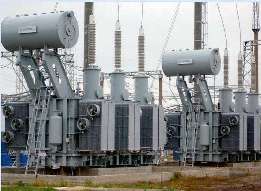
Izolyator 220kV bushings installed on Togliatti Transformer products
