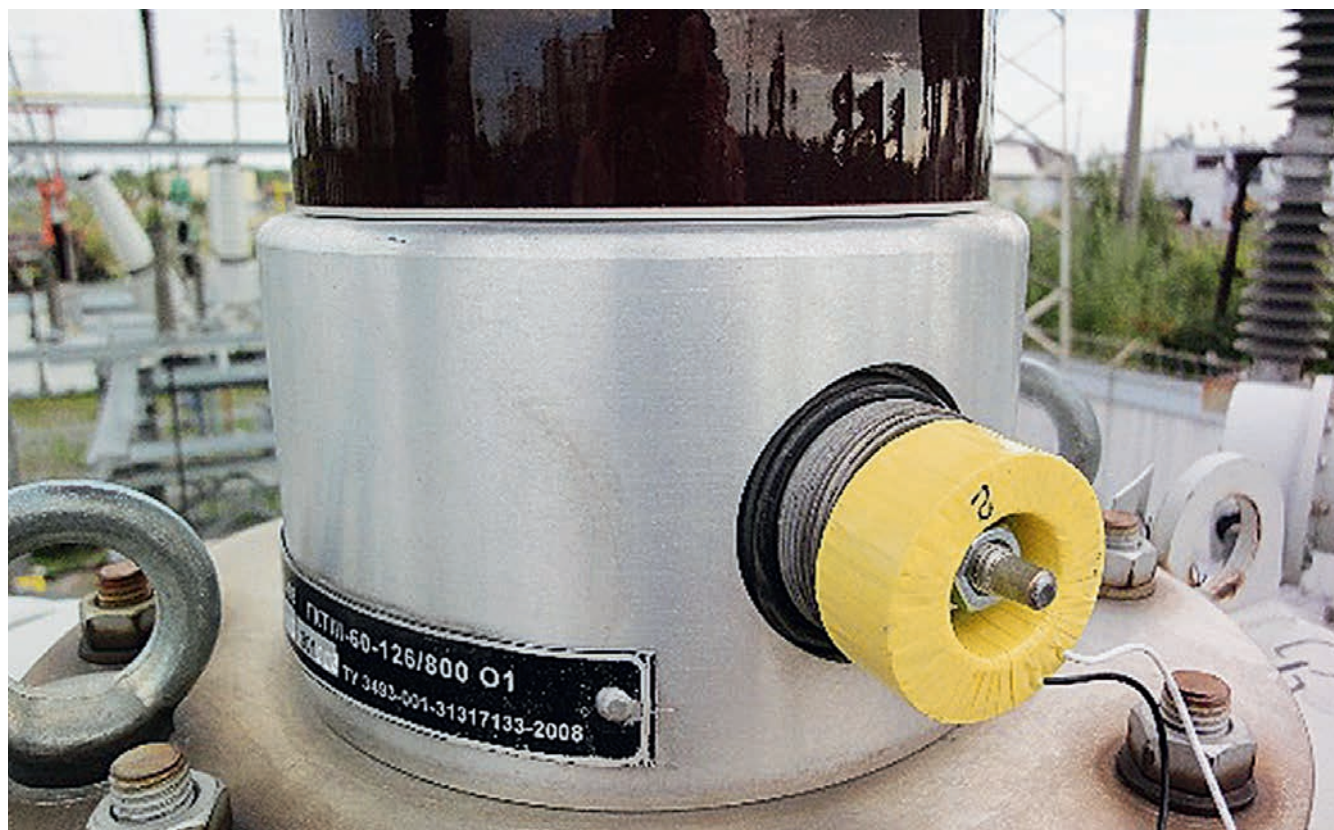
Construction design of the connecting device to the measuring tap with built-in current transformer
