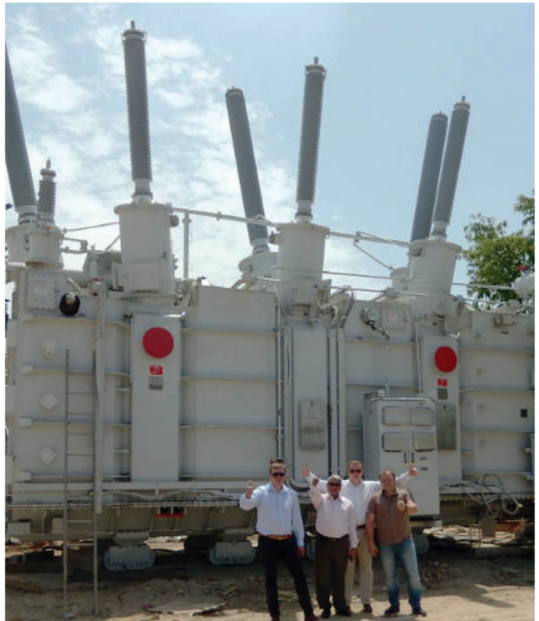
Supervision installation of Izolyator-made bushings at Bamnauli 400 kV substation in India is complete. Left to right: Andrey Shornikov, Dr. Ashok Singh, Ivan Panfilov and Dmitry Mashimistov
