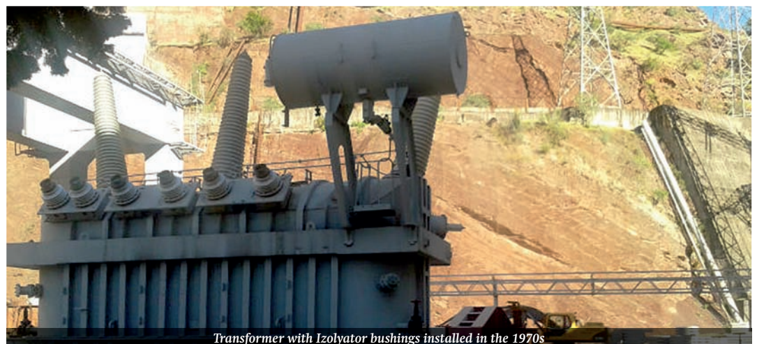
Transformer with Izolyator bushings installed in the 1970s
